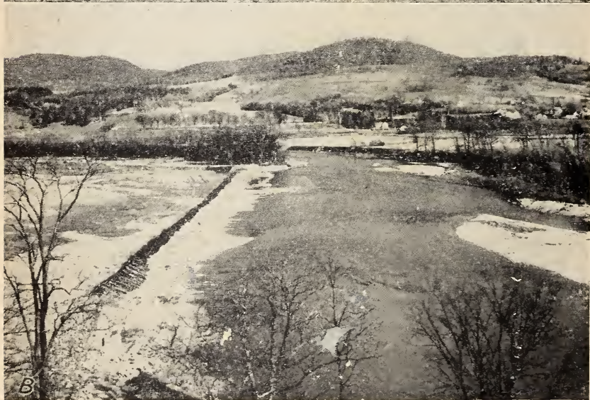
FIGURE 12.—Tree barricade across main chute. A , Trees are pushed into place by bulldozer and securely cabled together; B , completed structure showing rock-filled log crib at end (lower left).
